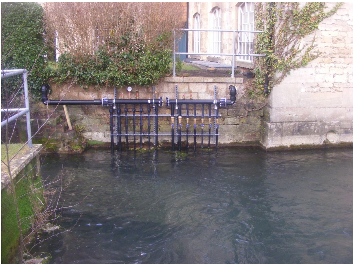
Figure 1: main flow and return manifolds for the FireFlo collector system with FireFlo panels submerged below
